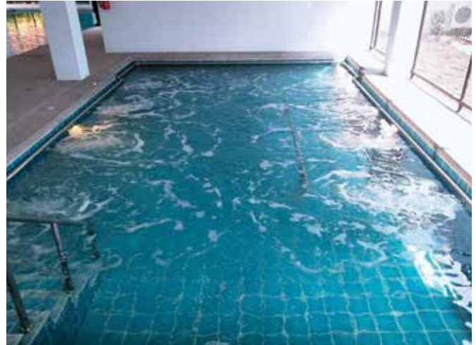
Waterco's Electroheat solution ensures the water temperature remains at a comfortable 37 °C
